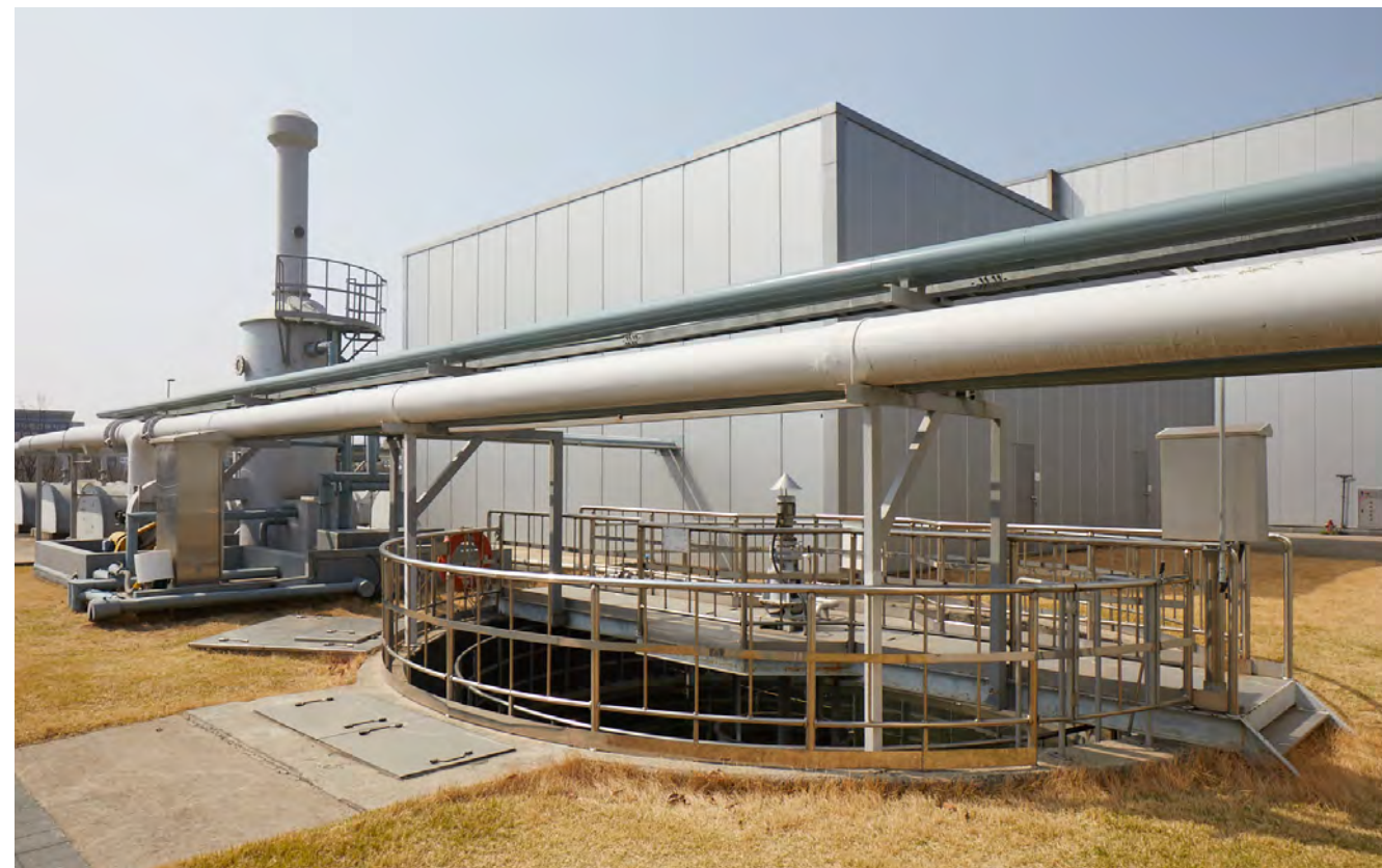
Beauty Park Osan's wastewater storage facilities
